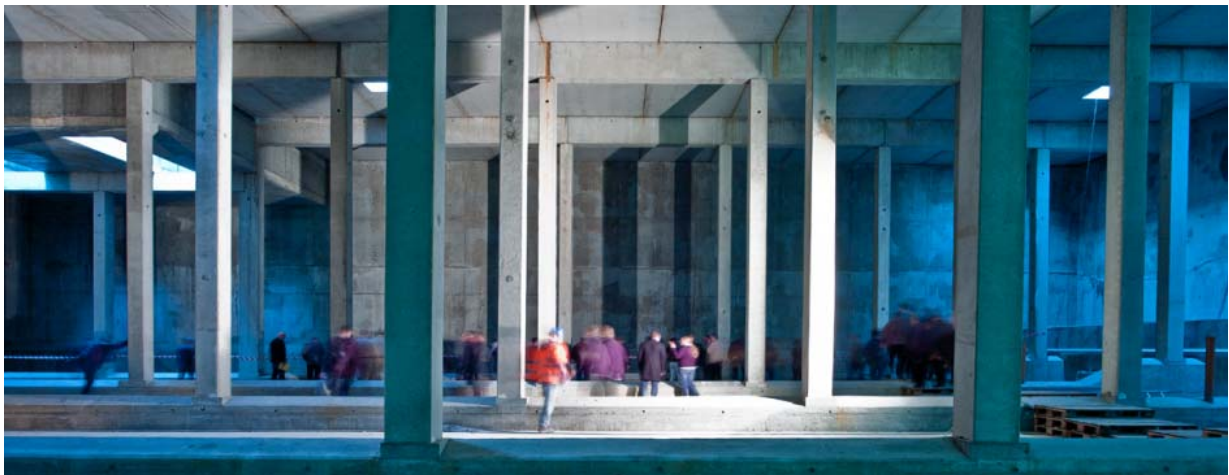
Figure 4 Interior of new CSO storage facility. Approximately 67,000 m 3 of new storage was built along with the real-time control system.
